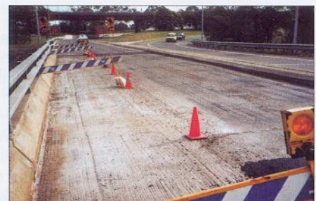
FIGURE 14 - SCABBLED BRIDGE DECK
