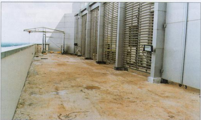
FIGURE 42 - EXPOSED CONCRETE ROOFTOP AFTER RADCON #7 TREATMENT
