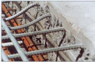
FIGURE 11 - EXPOSED CONSTRUCTION JOINT
